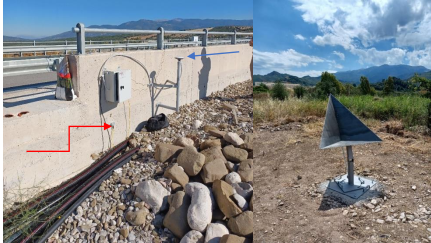
Figure 2: At the left: the 3D axis accelerometer and the low cost GNSS receiver that were installed at Asteri Dam. The red arrow shows the accelerometer while the blue one shows the GNSS antenna. The box contains all the other necessary equipment. At the right: Aluminum corner reflector installed in Patras University Campus.
